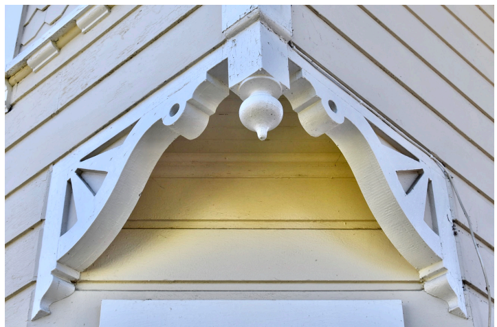
At right: Sunburst brackets with knob pendant in the corner of the bay window.
