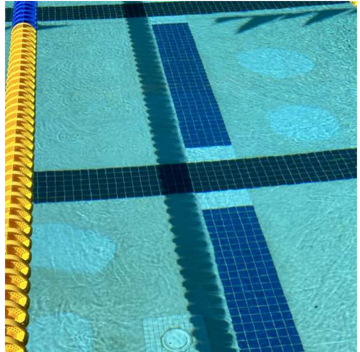
Image 22: Plaster Delaminating in 50-Meter Pool
