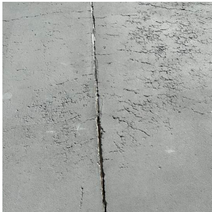
Image 18: Failing Pool Deck
