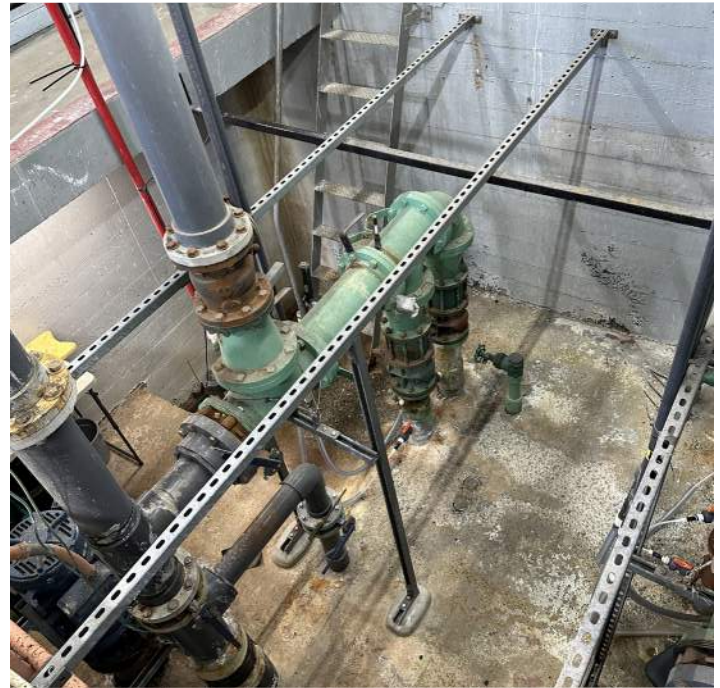
Image 2: Diving Pool Piping
