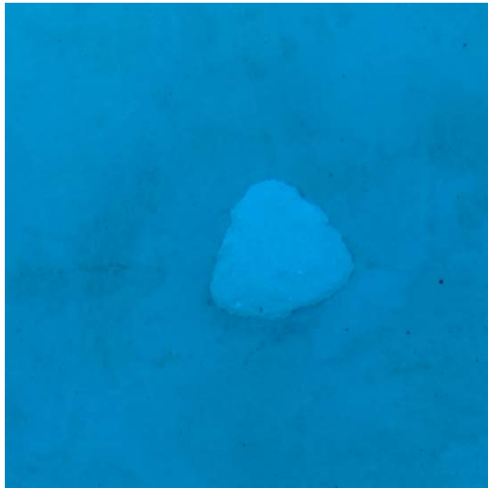
Image 16: Delaminating Plaster in Diving Pool
