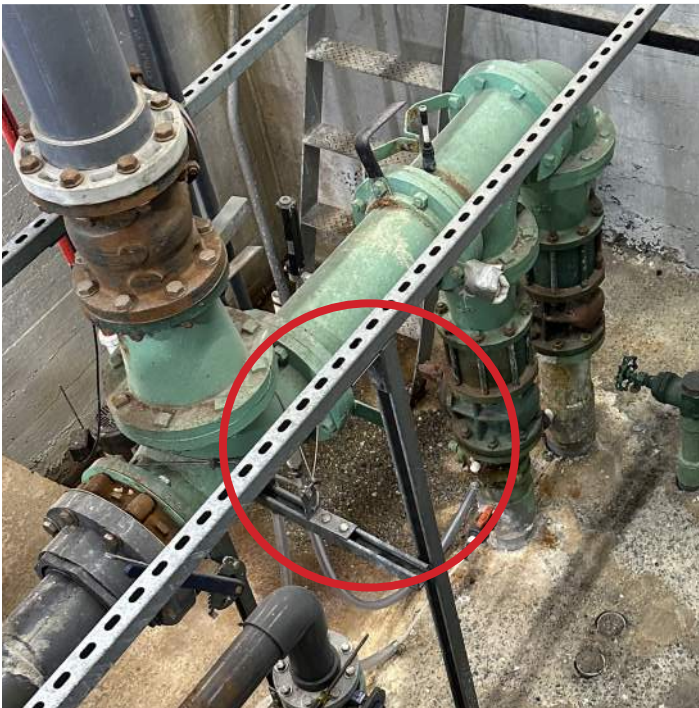
Image 21: Evidence of Leak in Pump Pit
