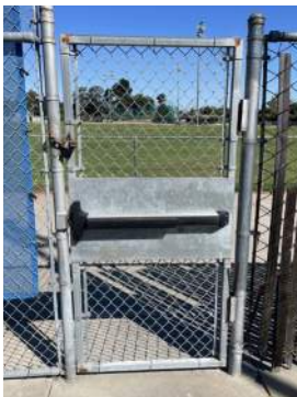
EXISTING CHAINED EXIT
