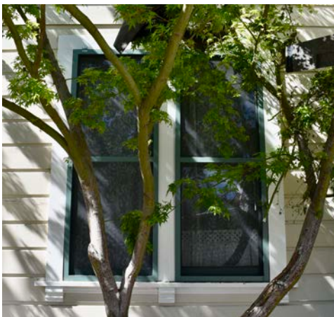
At left: Paired double-hung windows on the south side of the original first story of the rear block of the house.
