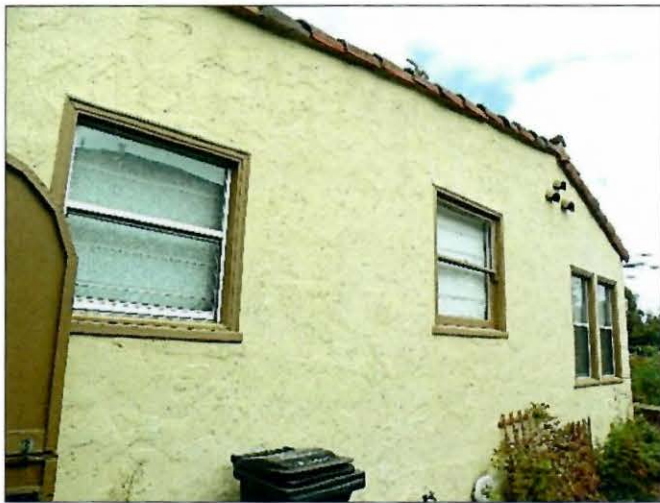
Photo No: 100_2719; View: S side-elevation from rear towards Main St. Photo Date: August, 2020; Camera Facing: NNE.
