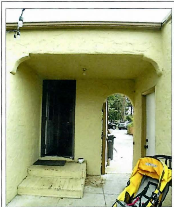
Photo No: 100_2717; View: Arcaded Wing Wall interior view looking out onto driveway. Photo Date: Sept., 2020; Camera Facing: NE.
