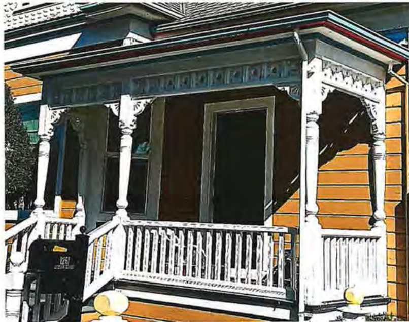
Photo No: IMG_7305; View: Front Porch: showing turned colonettes, carved brackets, Eastlake freize and balustrade. Photo Date: 2/6/2026; Camera Facing: NE.
