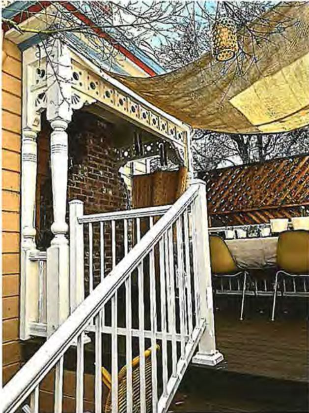
Photo No: IMG_1423; View: Side Porch showing original turned colonettes, carved brackets, and Eastlake block frieze. Along with altered entry with side ballustrade removed and new extended porch floor and new porch and entry stair railing. Photo Date: 2/6/2026; Camera Facing: SW.
