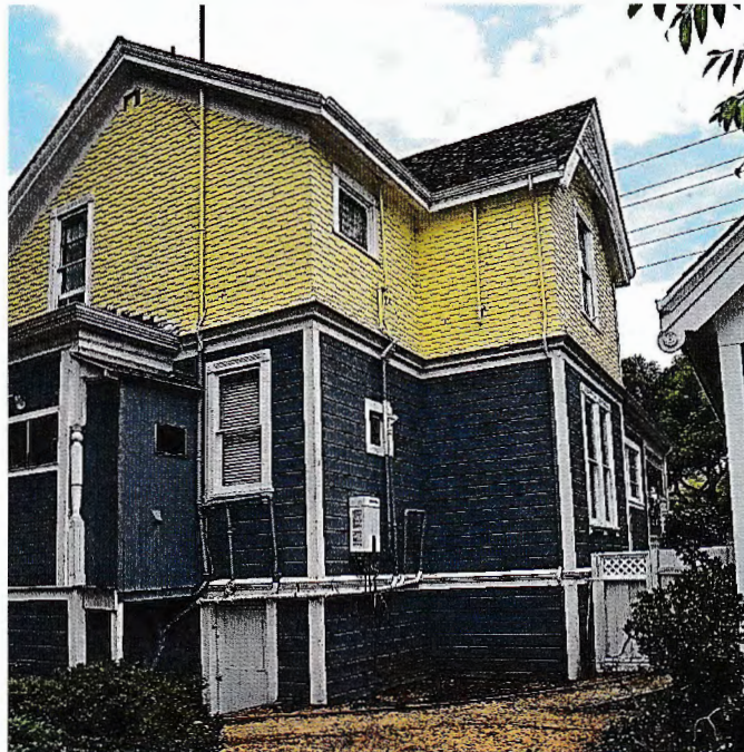
Photo No: 100_3656; View: Partial W side-elevation & partial rear façade. Photo Date: 8/2/2024; Camera Facing: E
