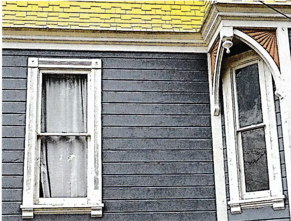
Photo No: 100_3647; View: Typical single dbl-hung window with fluted trim, corner blocks, brackets and cut-away bay window with sunburst brackets and drop pendant; Photo Date: 8/2/ 2024; Camera Facing: W.
