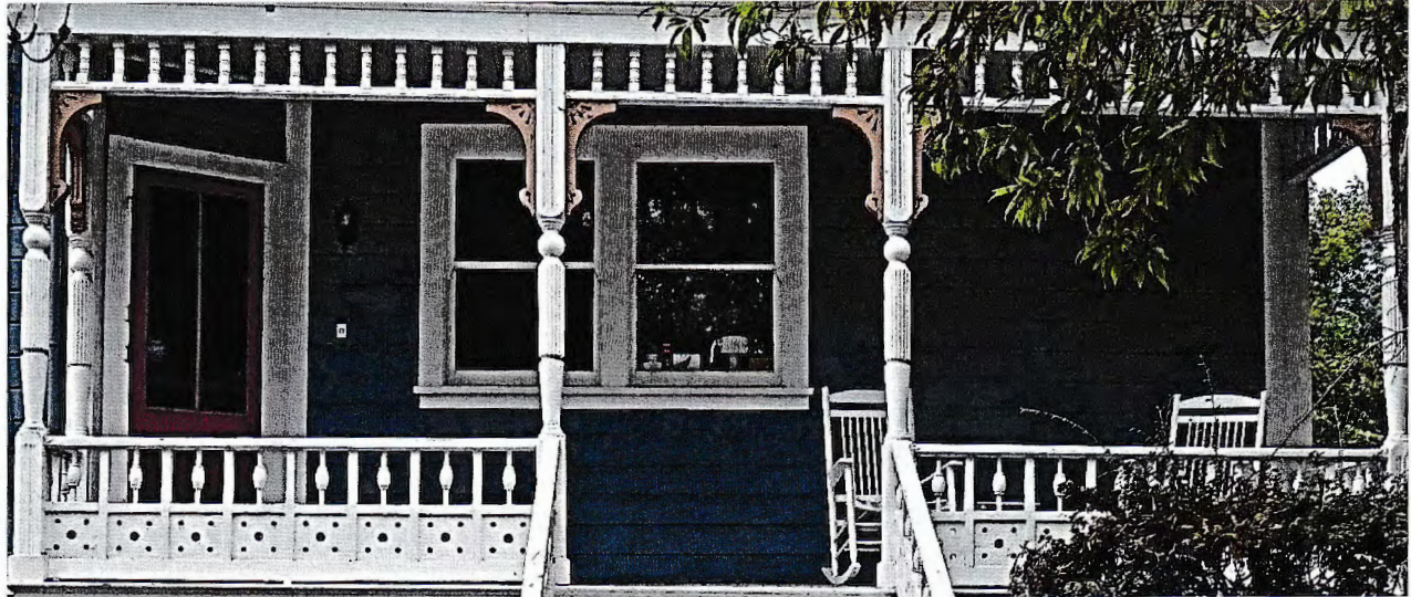
Photo No: 100_3643; View: Side Porch showing entry & ballustrade with Eastlake blocks; Photo Date: 8/2/2024; Camera Facing: SW.
