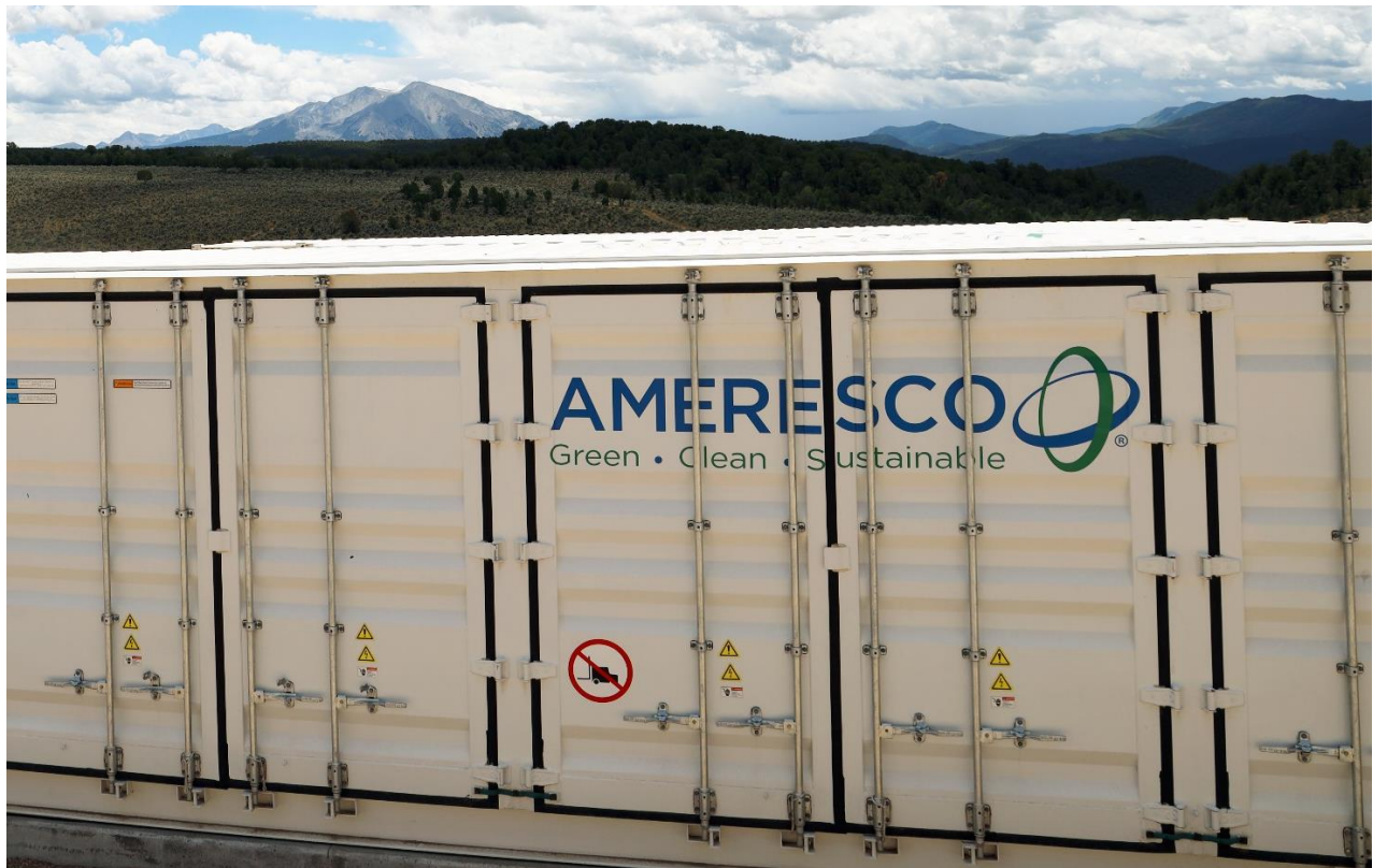
Example of a typical Battery Energy Storage System
