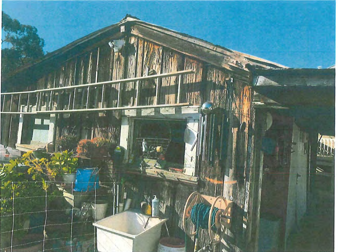
Front of the shed showing the various sizes of wood boards and condition of the shed.
