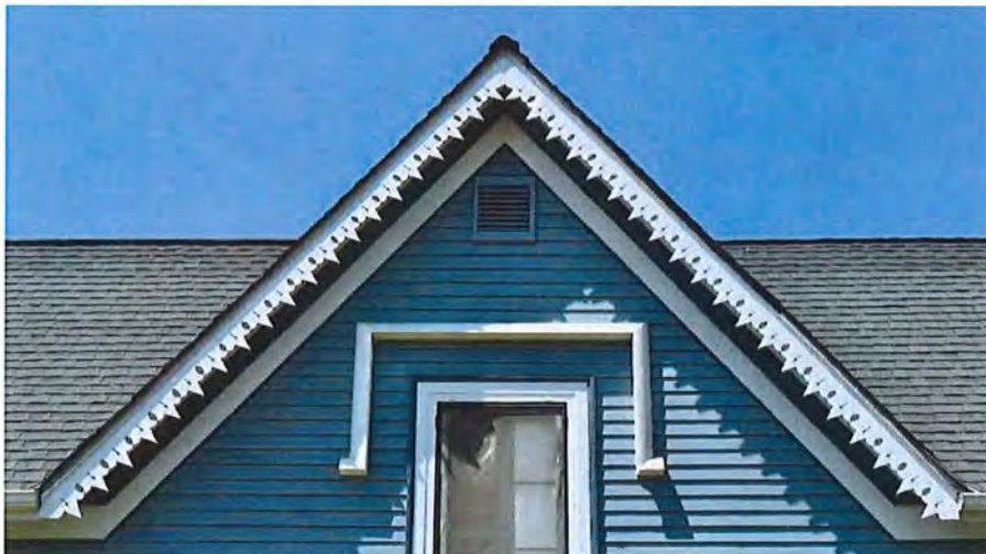
The front of the house with a detail of the bargeboard and the drip mold over the second story window.
