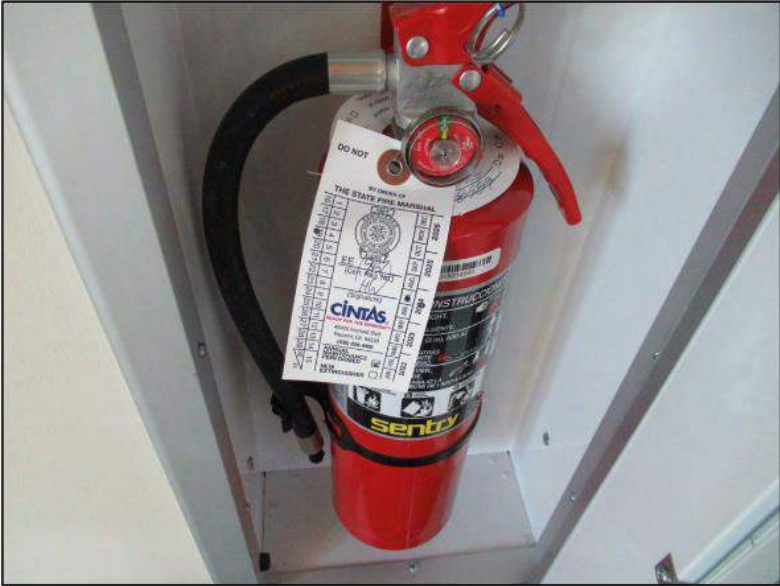
26. Fire extinguishers have current service tags.
