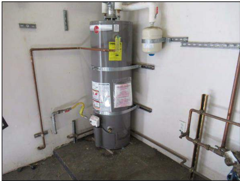
24. Domestic water heater is relatively new.
