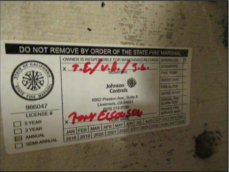
28. Five year fire sprinkler label is current.
