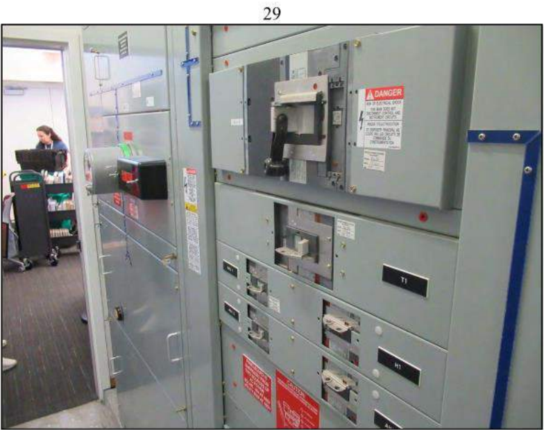
29. View of the 800-ampere main switchboard.
