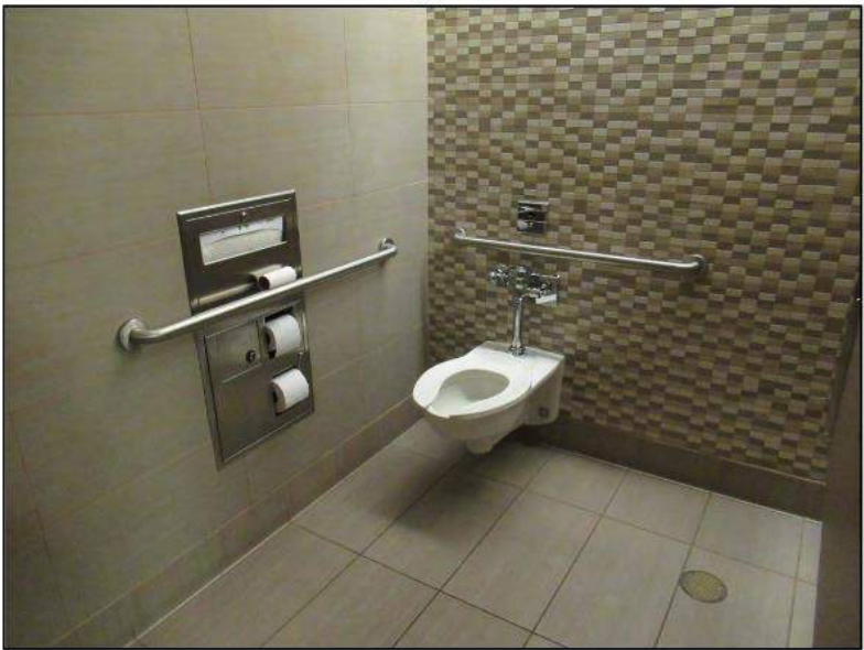
26. Toilets are wall-mounted with automatic flush valves.
