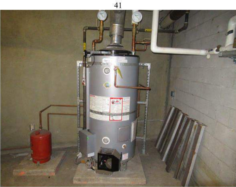
41. American Standard gas domestic water heater.
