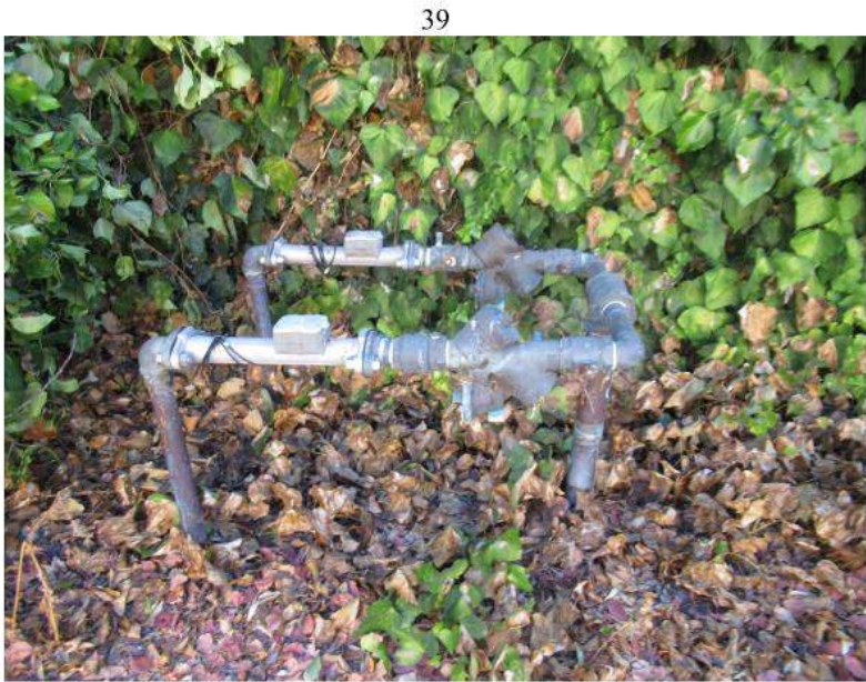
39. Main domestic and irrigation water assembly.
