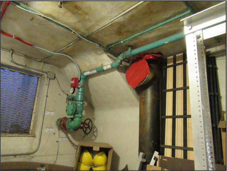
27. Fire sprinkler assembly in the basement.
