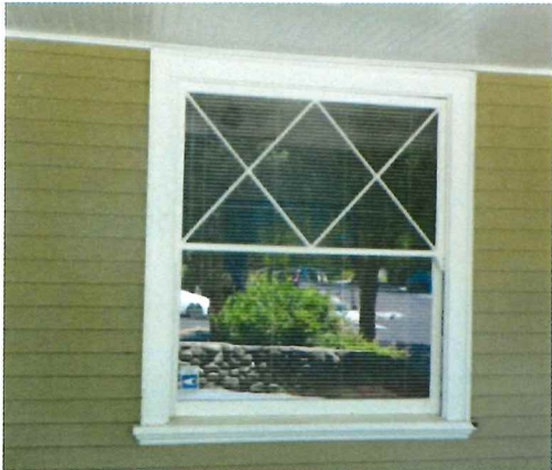
Photo No: 100_2374 View: First story window with distinctive diamond shaped panes with crossed muntins in upper sash. Photo Date: May, 2018; Camera Facing: NE
