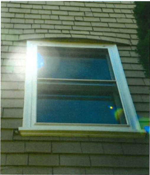
Photo No: 100_2348 View: North side-elevation 2nd story window with curved row of shingles over the top of the window trim. Photo Date: May, 2018; Camera Facing: SE
