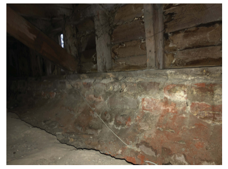
PHOTO OF DETERIORATING INNER COURSE OF BRICK FOUNDATION 1
