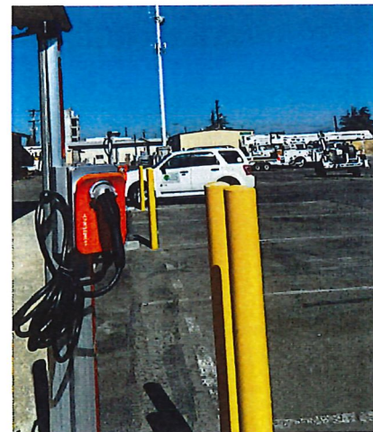
Level 2 EV Chargers at Utility Yard
