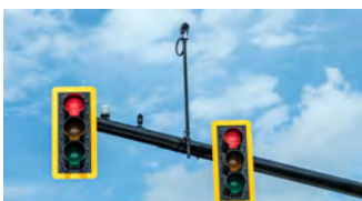
Replace Roadside Pole Mounted Signal Heads with Overhead Signal Heads
