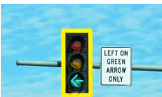
Protected Left-Turn Phase
