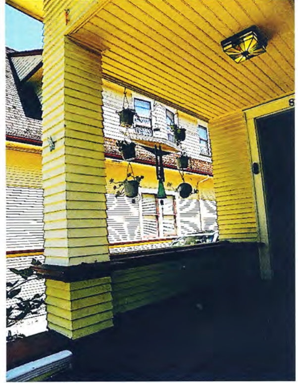
Photo No: 100_3237 View: Front porch view of open side, support column & knee wall Photo Date: 8/18/2023; Camera Facing: NE
