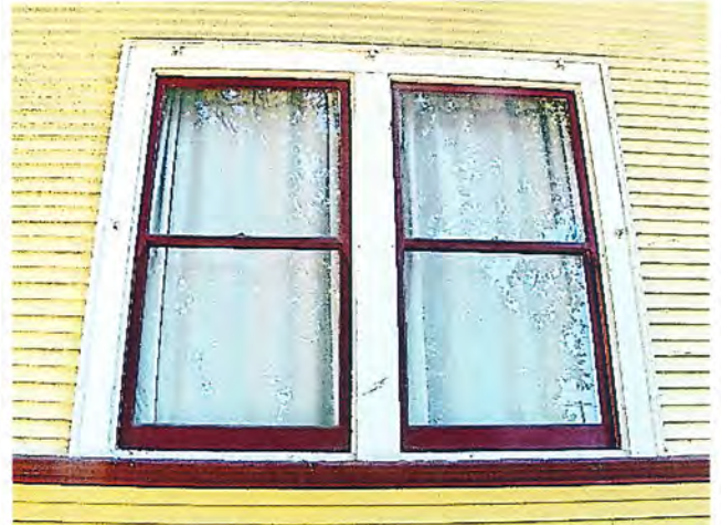
Photo No: 100_3244 View: Front façade's first story pair of windows with back-banded trim abutting water table molding. Photo Date: 8/18/2023; Camera Facing: E
