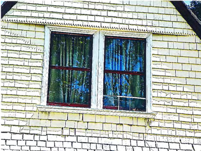
Photo No: 100_3286 View: Front Gable face windows showing the row of shingles & sawtooth shingles that curve over it. Photo Date: 8/18/2023; Camera Facing: E
