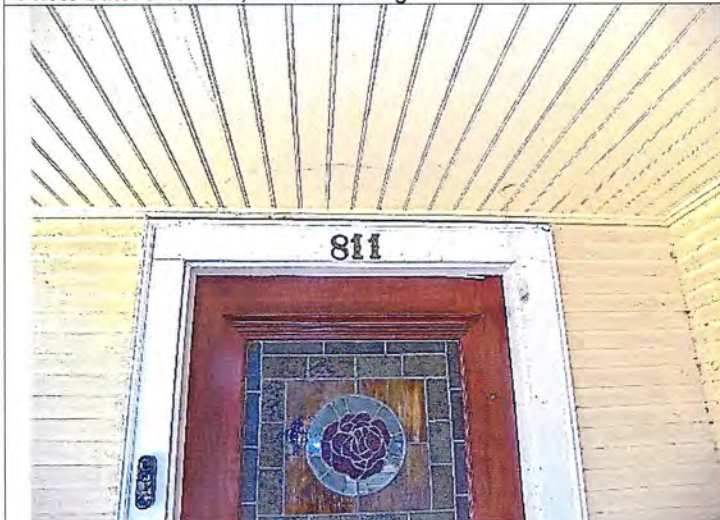
Photo No: 100_3242 View: Front porch beadboard ceiling & narrow vertical wall sheathing Photo Date: 8/18/2023; Camera Facing: E
