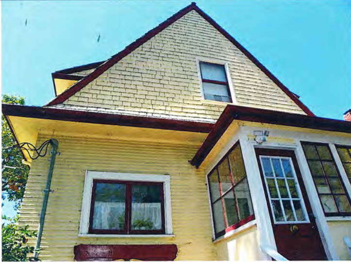
Photo No: 100_3263 View: Rear Façade showing rear gable Photo Date: 8/18/2023; Camera Facing: W
