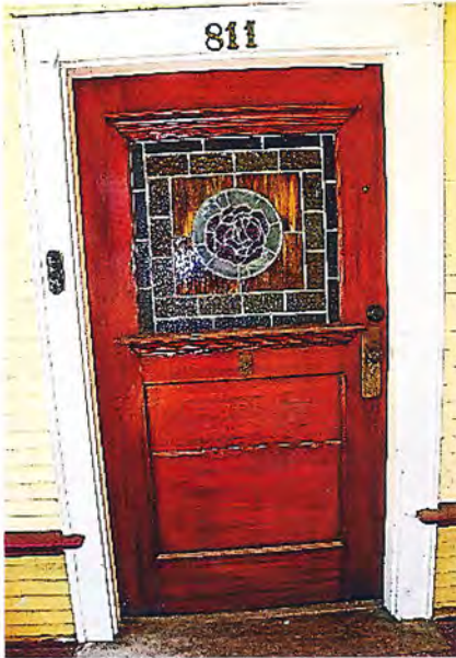
Photo No: 100_3240 View: Front Door with back-banded door trim Photo Date: 8/18/2023; Camera Facing: E
