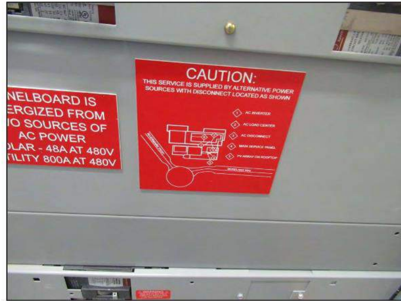
27. The electrical service is supplemented by a solar system.
