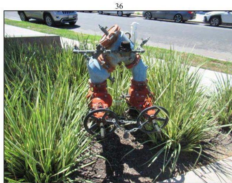
36. View of the 6" fire water service at Rivermark Pkwy.
