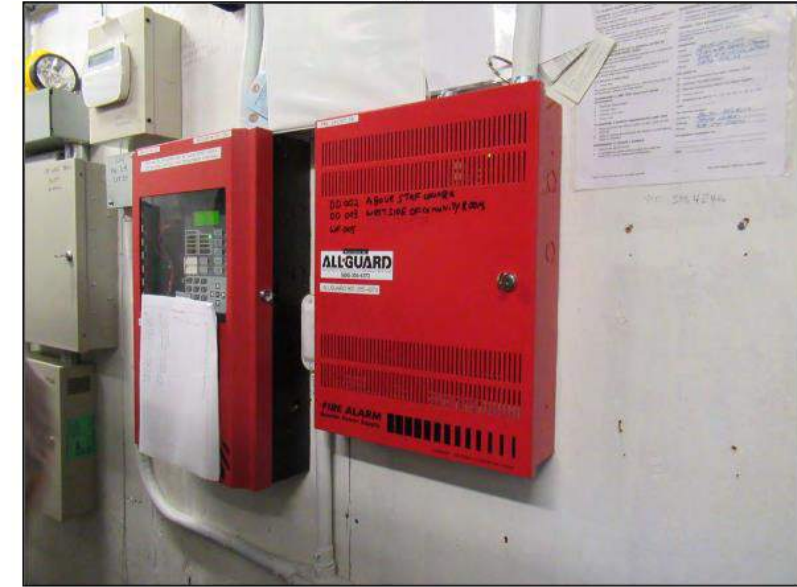
33. View of the Edwards fire alarm control panel.
