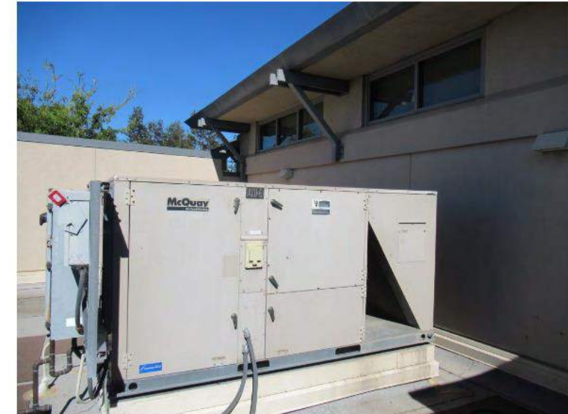
38. One of four McQuay packaged units.
