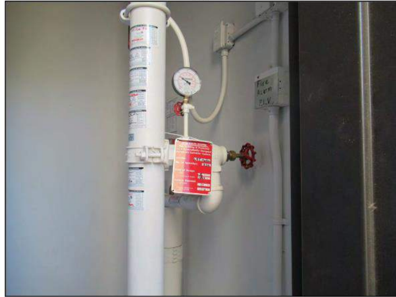
31. Incoming fire water service is to a 4" riser.
