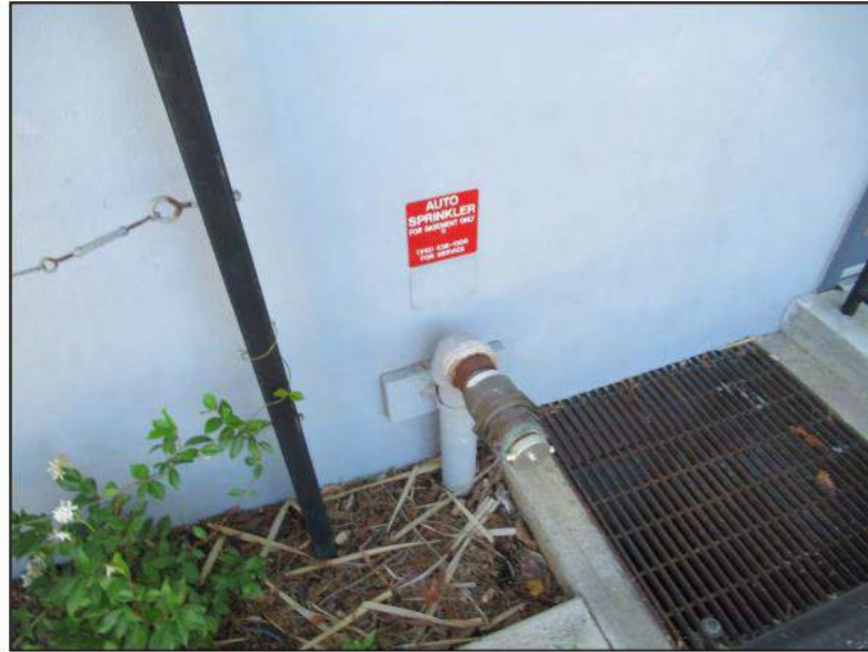
25. Incoming 2" galvanized steel water service for fire sprinklers in basement.
