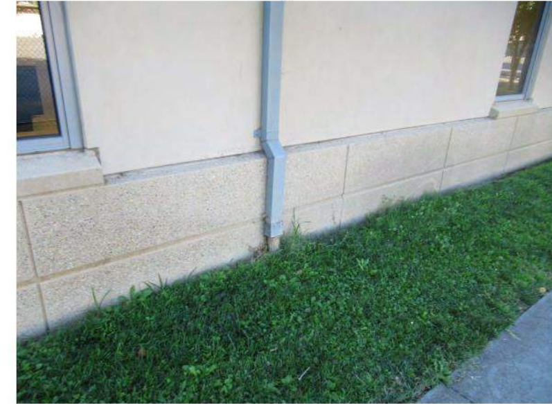
13. Downspouts connect to the underground collection piping.
