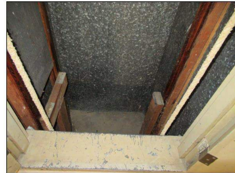
4. Manual dumb waiter to the basement.
