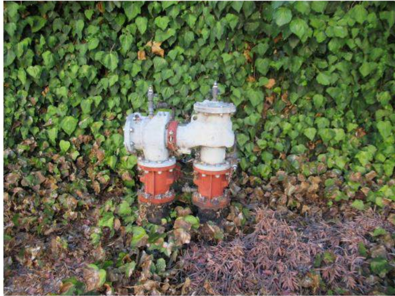
47. Main fire water service on the east side of the site.
