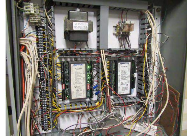
37. Alerton energy management system (EMS).
