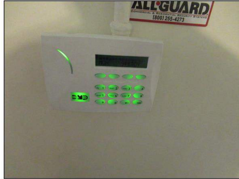
29. Remote fire alarm panel.
