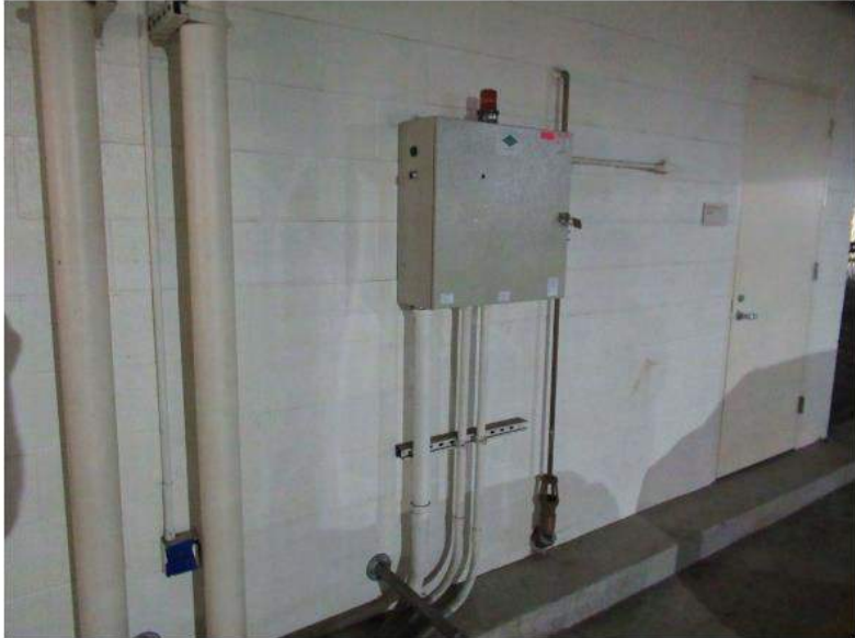
40. Controller for one of the sump pumps in the garage level.
