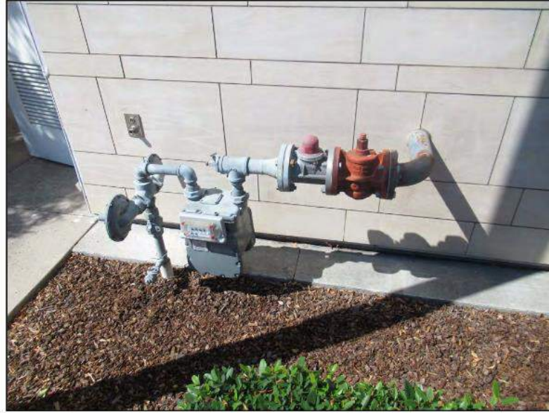
23. Gas service with seismic valve.
