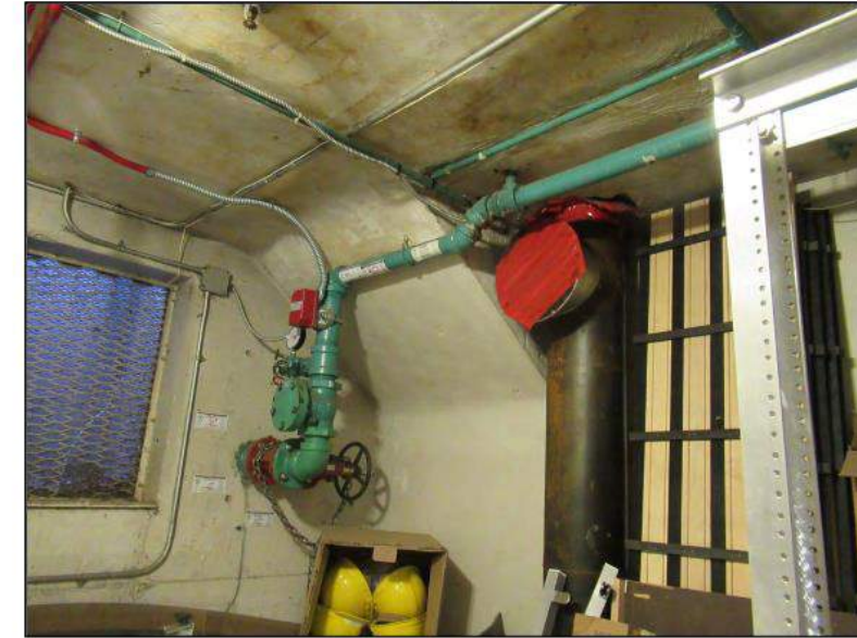
27. Fire sprinkler assembly in the basement.
