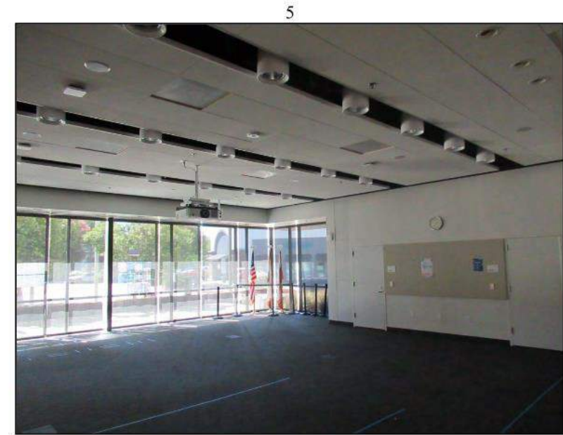
5. Conference room has a water intrusion issue that is under investigation.
