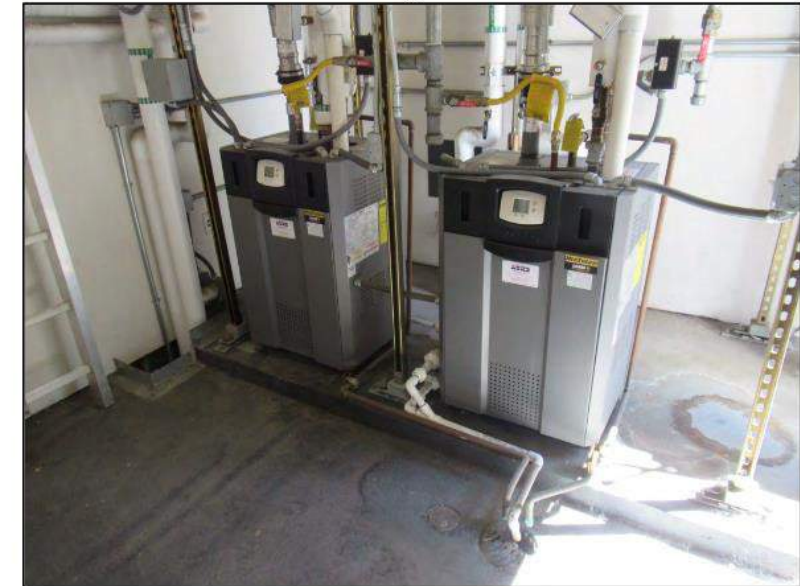
18. Natural gas-fired boilers for space heat.
