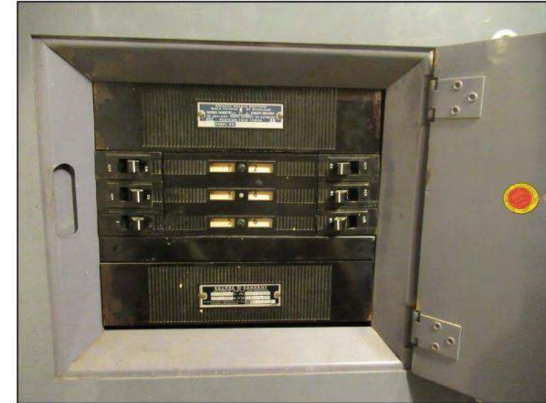
23. Original 1955 Square D panelboard.
