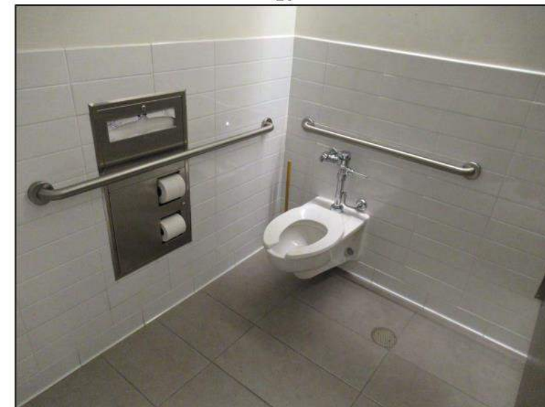
20. Toilets are wall mounted with manual flush valves.
