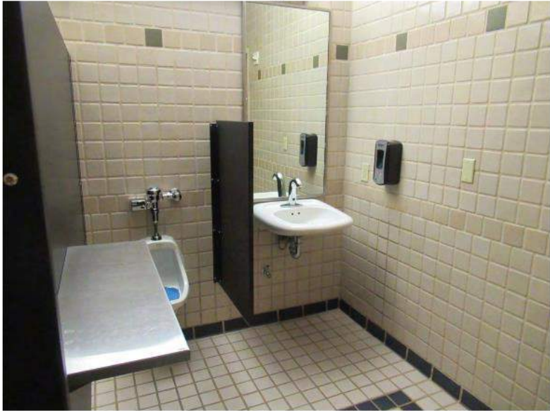
43. Lavatories have automatic faucets and urinals have automatic flush valves.
