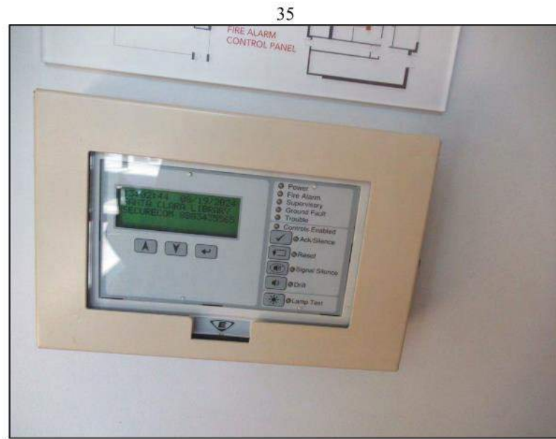
35. Remote fire alarm device in the main lobby.
