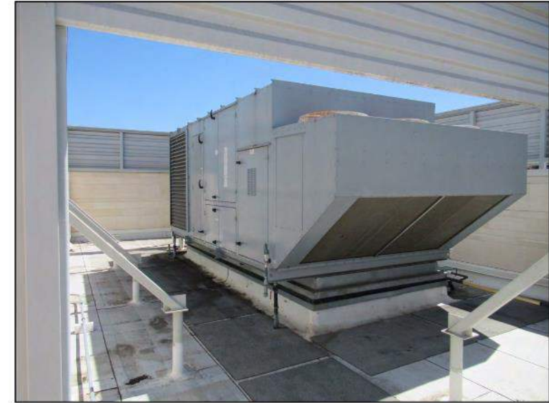
21. One of two 20-ton packaged Airtex units. Number two unit is down for repairs.
