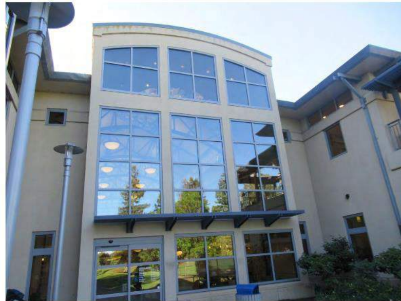
12. View of the window wall on the northwest corner of the building.
