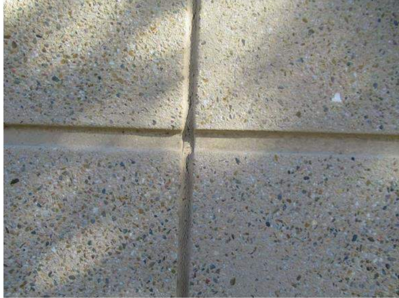
15. Caulking at the precast panel joints is shrinking and needs to be cut out and replaced.
