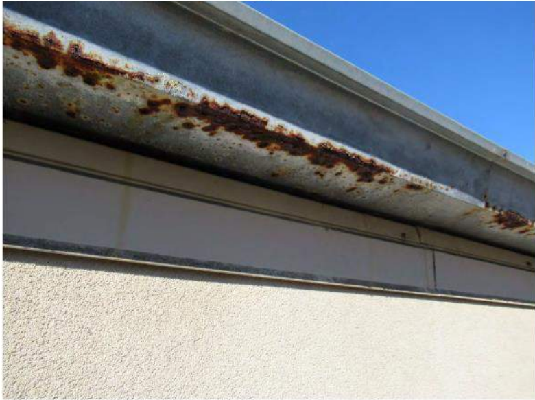
27. Flashing on the northeast mechanical well is deteriorating.
