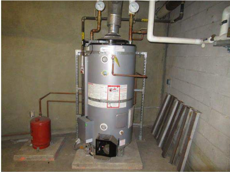
41. American Standard gas domestic water heater.
