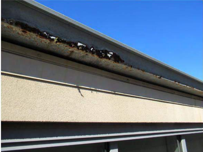
28. Flashing on the northeast mechanical well is deteriorating.
