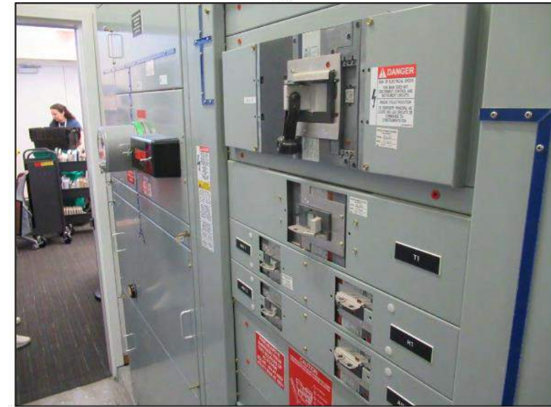
29. View of the 800-ampere main switchboard.
