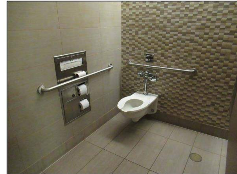
26. Toilets are wall-mounted with automatic flush valves.
