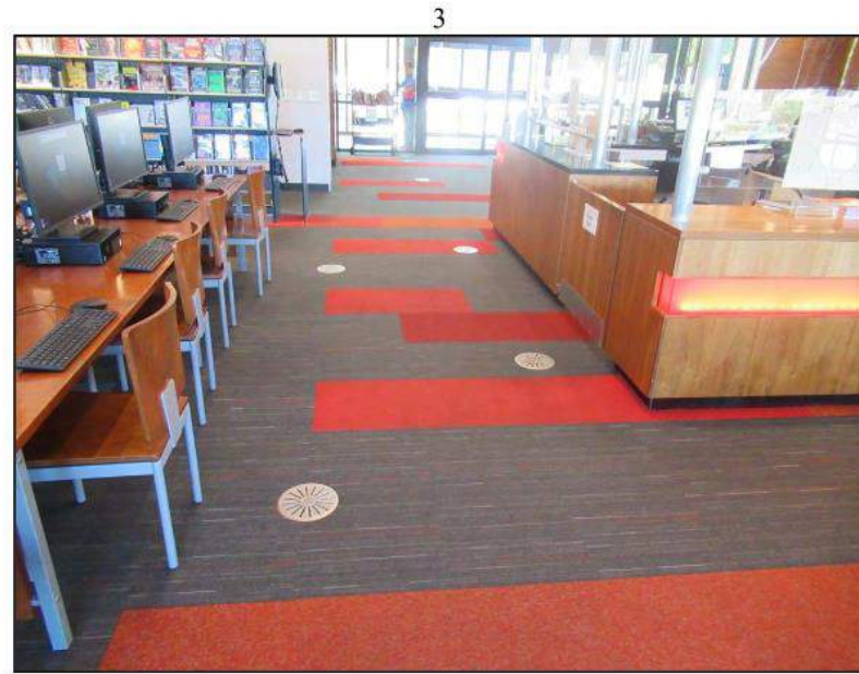
3. The entire floor area is raised flooring with vents for air circulation.
