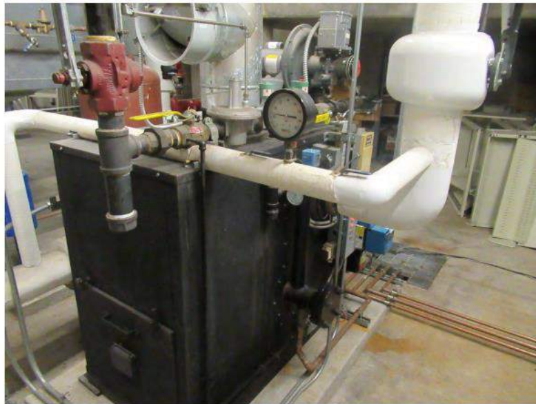
36. One of two Parker boilers for space heating.
