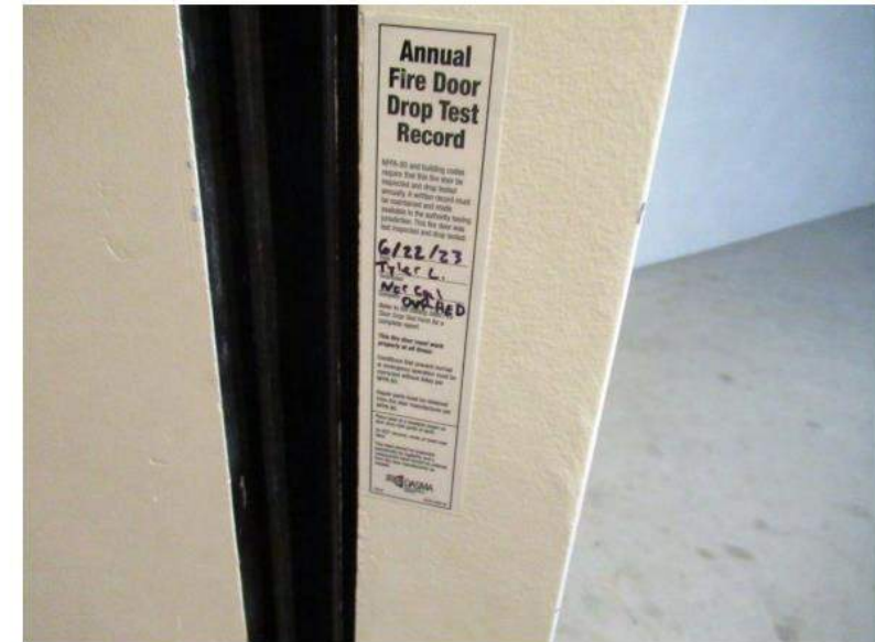
50. One of five fire doors that are regularly inspected.
