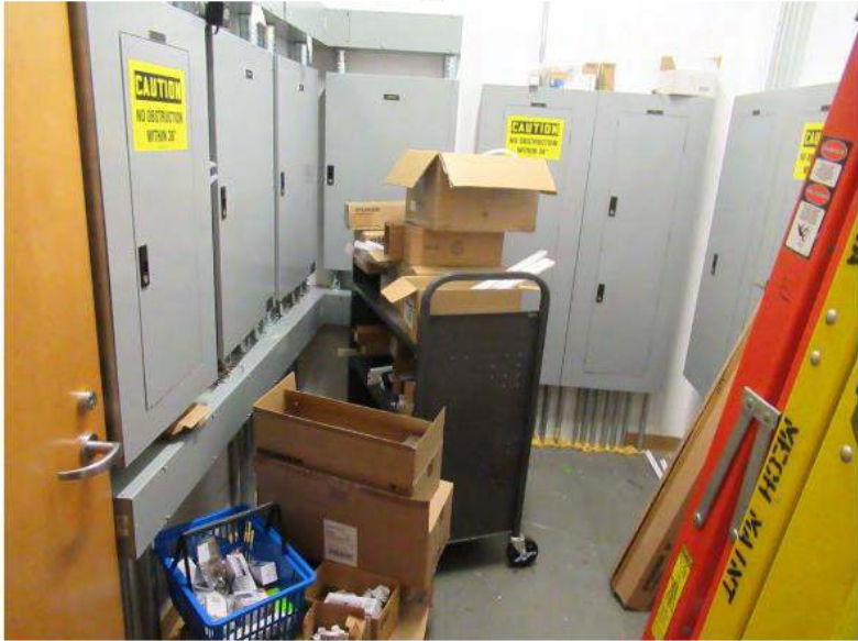
45. Several of the electrical rooms have storage that should be removed.
