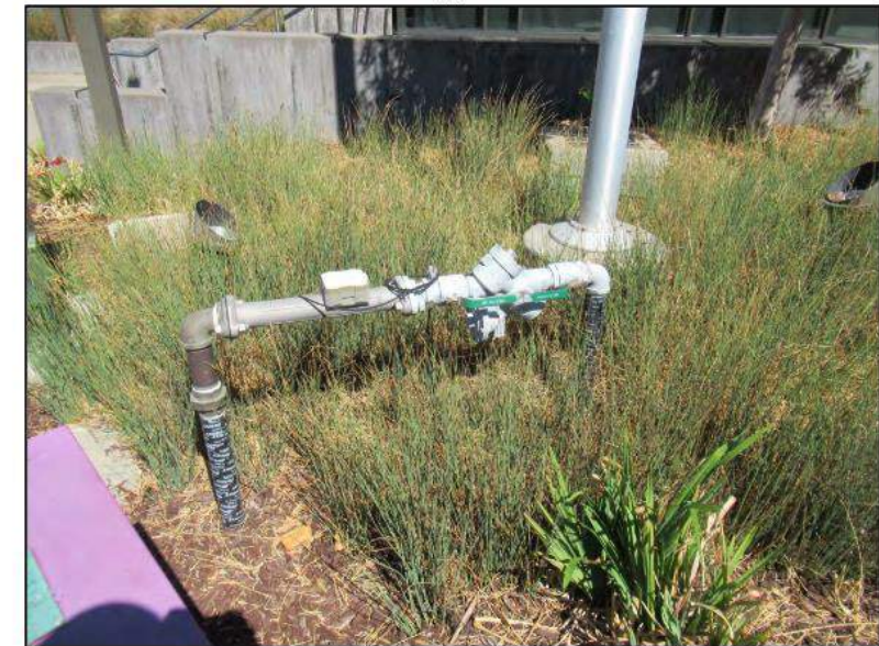
22. Incoming domestic water service.
