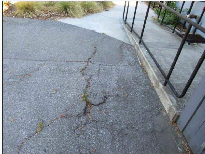
6. Damaged asphalt paving adjacent to the south employee entrance.
