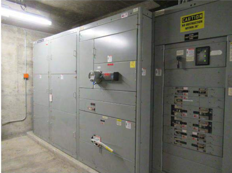
44. The main switchboard in the garage level is rated 2,000-amperes.
