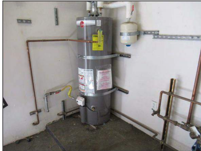
24. Domestic water heater is relatively new.
