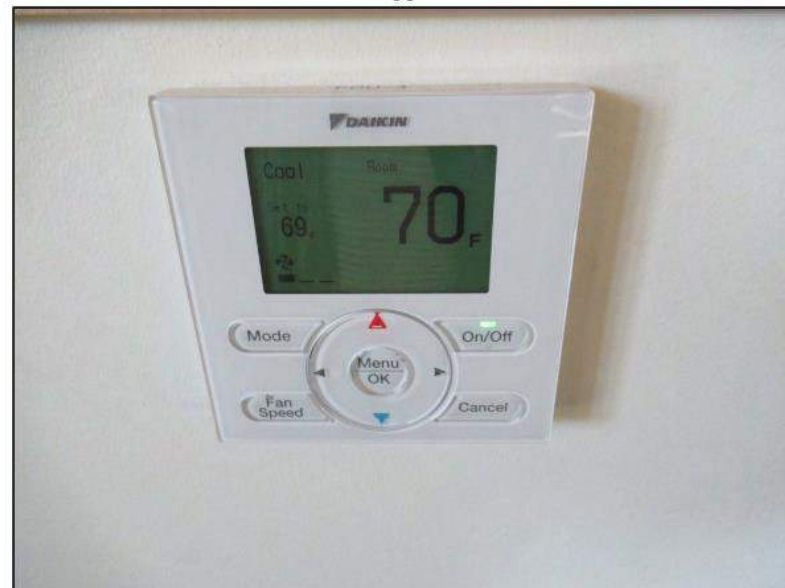
16. Daikin thermostat is controlled by the Daikin EMS.
