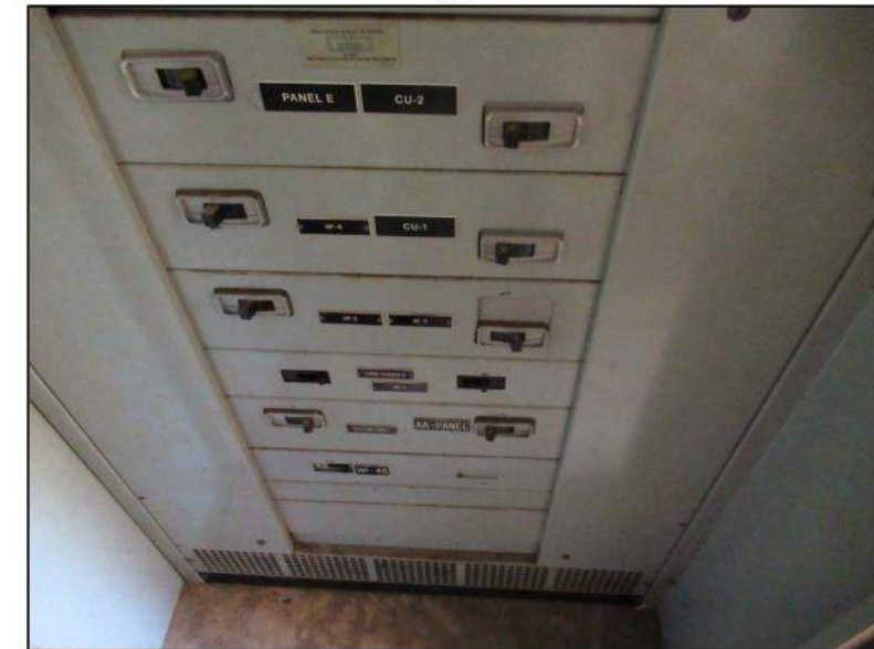
24. Main switchboard was installed in 2000.
