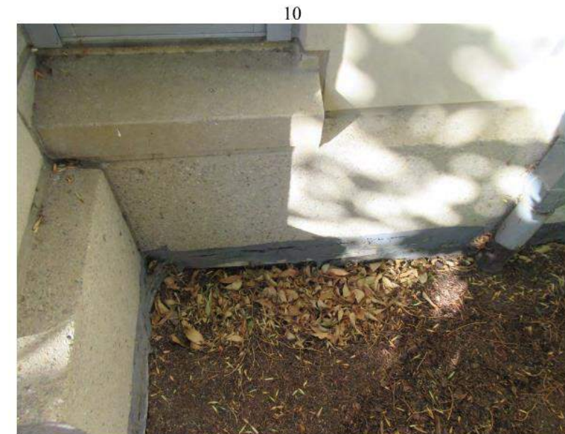
10. Sealant at the base of the building is shrinking.
