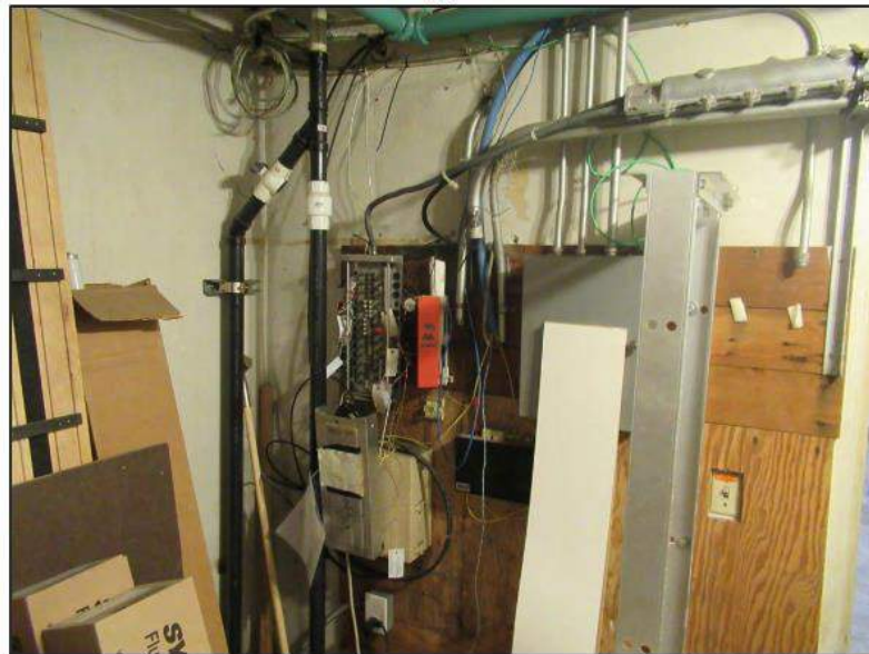
22. Telephone backboard in located in the basement.
