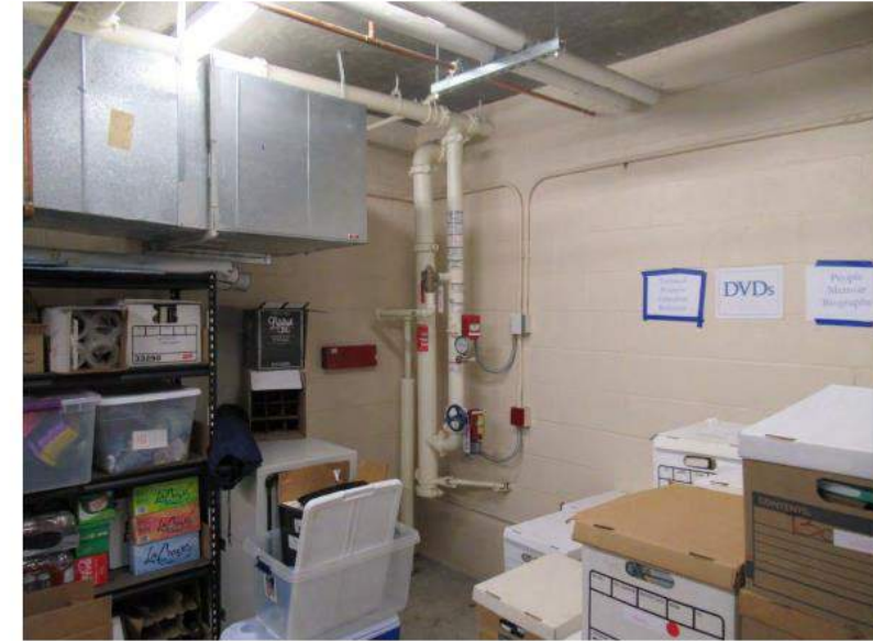
49. One of five fire sprinkler risers in the building.
