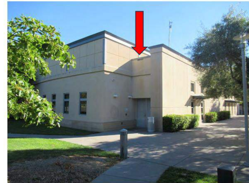
14. View of the southwest corner. Note staining from the roof scupper above door.
