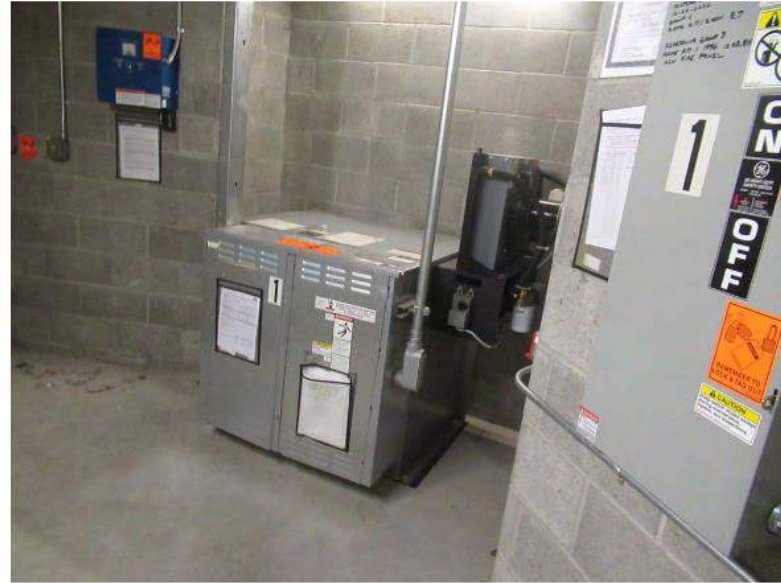
51. One of three hydraulic elevator machines.
