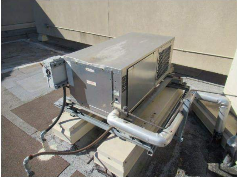
30. One of several condensing units that serve the server rooms.
