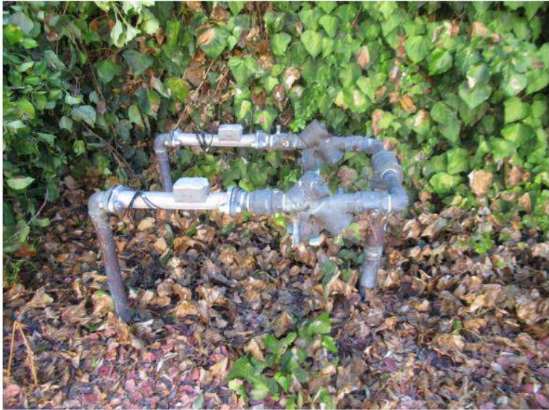
39. Main domestic and irrigation water assembly.
