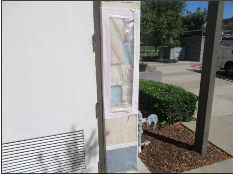
11. Exterior stone cladding is a subject of an ongoing investigation.
