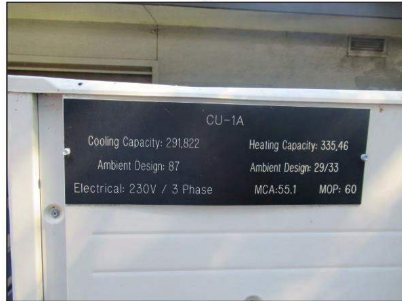
15. Air -cooled condensing units have service labels.
