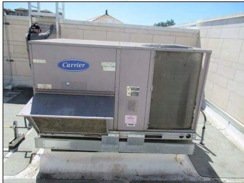
20. One Carrier 5-ton packaged unit on the roof for the community room.
