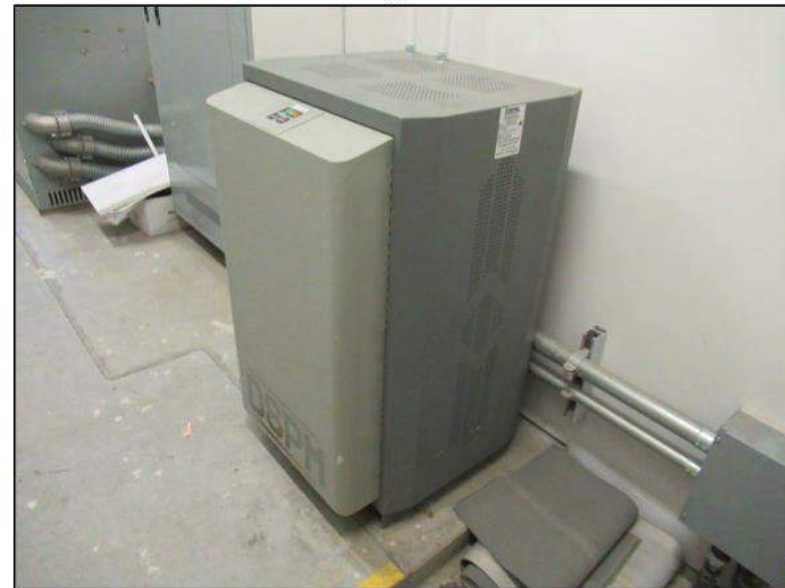
28. An Inverter supplies backup power to emergency egress lighting.
