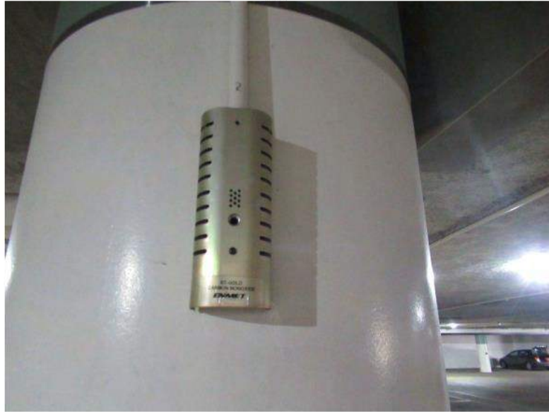
35. Carbon Monoxide sensors in the garage activated the exhaust system.
