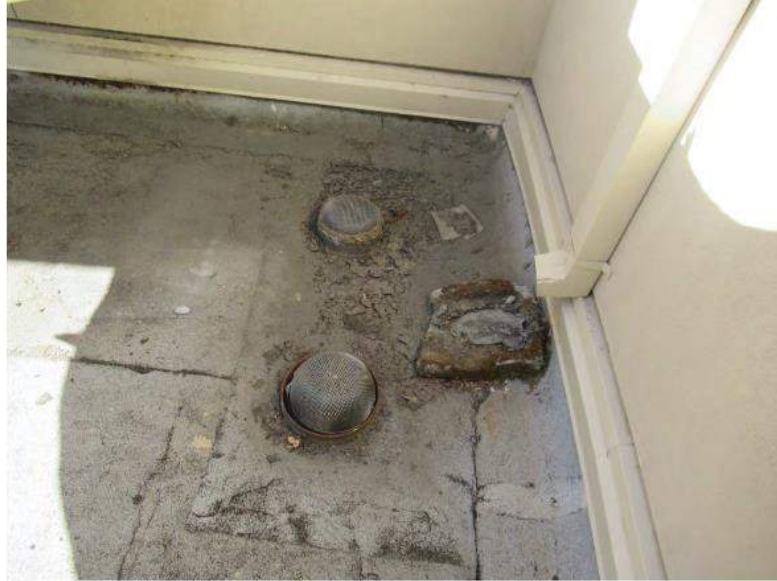
23. Roof drain wells are impacted with dirt and debris.
