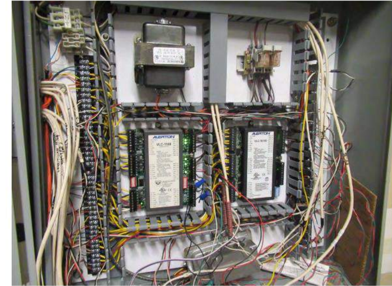
37. Alerton energy management system (EMS).
