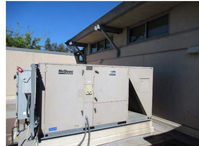
38. One of four McQuay packaged units.
