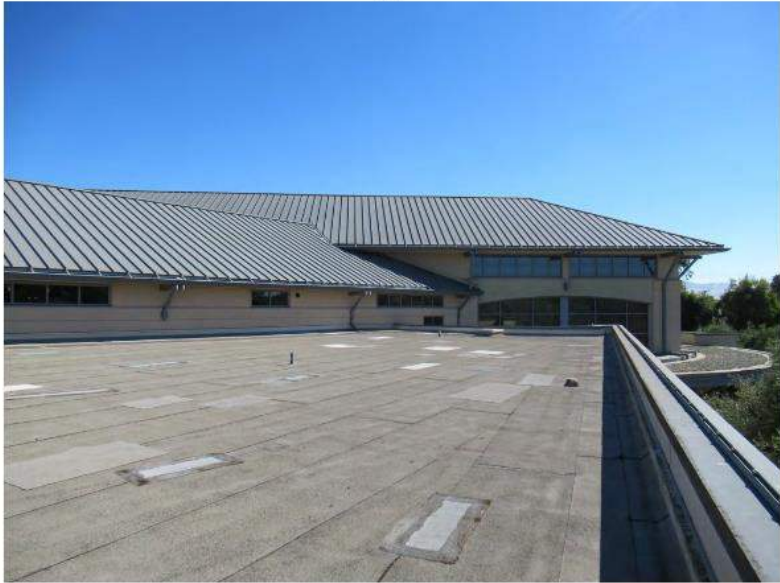
29. Roof membrane over the south roof is a multi-ply with capsheet that is 20 years old.
