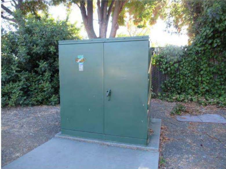
46. The Silicon Valley Power pad-mount transformer is rated 1,000kVA.
