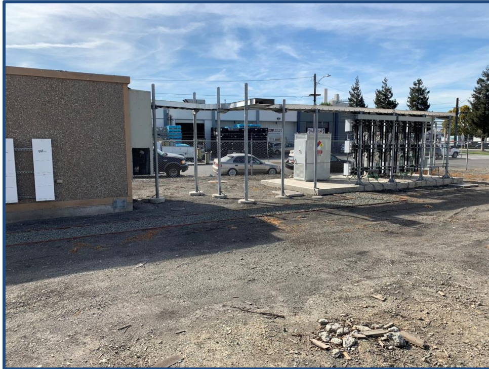
View of the existing electrical equipment on the subject (we have appraised the land only)
