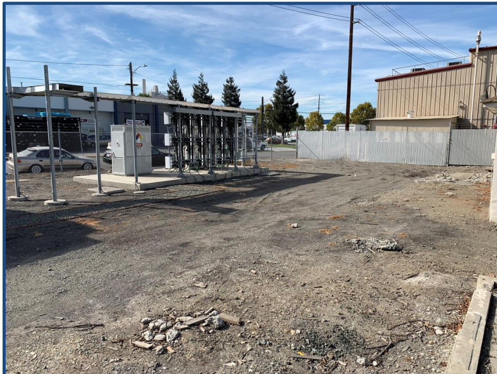
View of the subject looking towards the southwest corner of the property
