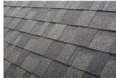
ROOF: SHINGLES (NEW COLOR) IN DARK GRAY COLOR ALL AROUND NEW HOUSES
