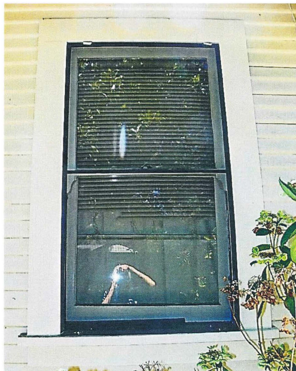
Photo No: 100_3089 View: Typical I-over-1 double hung window; August, 2022; Camera Facing: SSE
