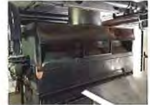
Swim Center Boiler
