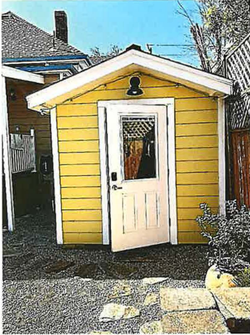
Above: Photo No: IMG_1414; View: “Original” Garage Rear façade and entry door seen from rear yard; Photo Date: 2/6/2026; Camera Facing: WSW.
