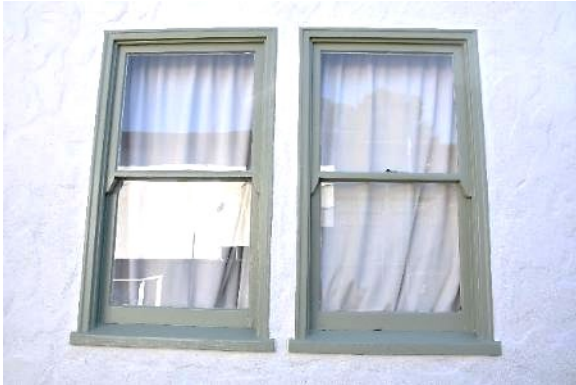
Figure 16. Views of original wood windows to be removed to accommodate new addition (above) and view of original wood window to be removed and opening enlarged to accommodate new sliding door (right).
