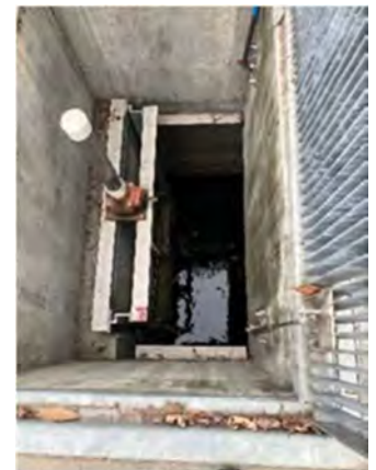
Storm Drain Slide Gate
