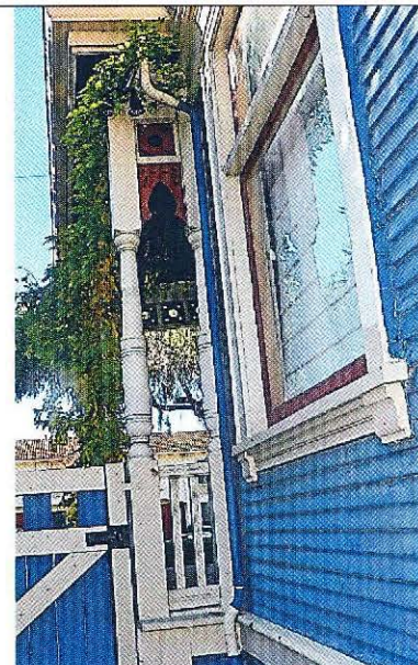
Photo No: 100_3433 View: Exterior rear of side porch towards street from driveway showing 1 full column & 1 Eastlake block; Photo Date: December, 2023; Camera Facing: WSW.
