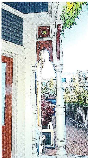
Photo No: 100_3360 View: Interior rear porch looking toward garage showing 1 full and 1/2 column and 1 Eastlake block; Photo Date: December, 2023; Camera Facing: E
