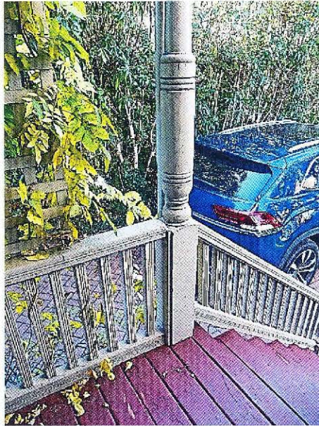
Photo No: 100_3374 View: Side porch balustrade & column base Photo Date: December, 2023; Camera Facing: S
