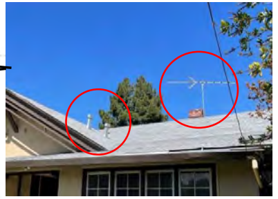
Phase: Design/Construction Comments: Add note. Remove TV antenna and exhaust vents from front of house. Vents to be relocated to rear elevation.
