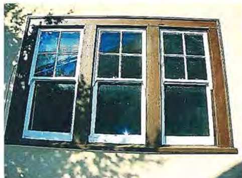
Above: Photo No: 100_2924 View: S side-elevation ribbon of 3 double-hung windows; Photo Date: December, 2021; Camera Facing: NNW
