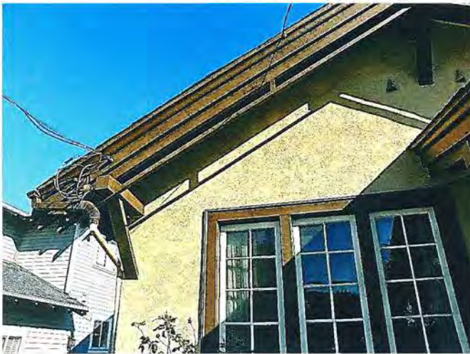
Photo No: 100_2896; View: Verge board on rake eave (Front); Photo Date: December, 2021 Camera Facing: ENE
