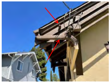
Phase: Construction Comments: Downspouts should not extend past bargeboard. Run downspouts inside of bargeboard. Remove excess electrical equipment.
