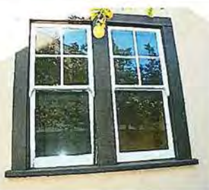
Left: Photo No: 100_2005 View: S side-elevation pair of dbl-hung windows (original); Photo Date: December, 2021; Camera Facing: NNW
