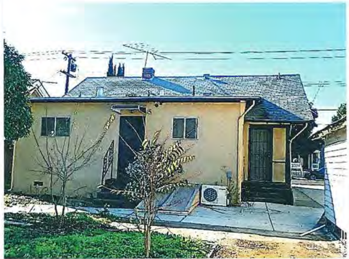
Photo No: 100_2909 View: Rear façade, view towards street; Photo Date: December 2021; Camera Facing: WSW
