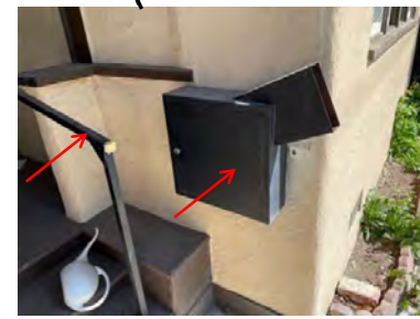
Phase: Design/Construction Comments: Adjust note. Remove handrail and mailbox. Patch stucco as needed.
