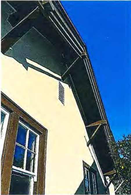
Photo No: 100_2916 View: S Side Gable, unenclosed eaves and knee braces; Photo Date: December, 2021; Camera Facing: NNE
