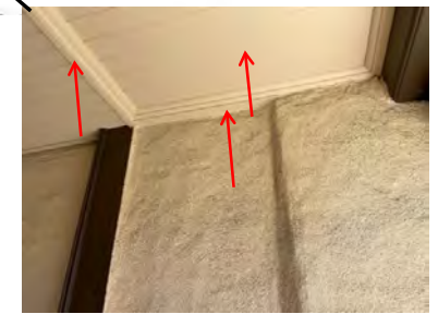
Phase: Pre-construction Comments: The porch ceiling height and trim varies. During construction, evaluate structure and conditions. Retain the bead board and crown at front of porch.
