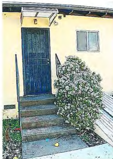
Photo No: 100_3005 View: Rear entry – (addition); Photo Date: December, 2021 Camera Facing: W
