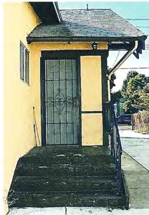
Photo No: 100_2921 View: Rear entry (believed original); Photo Date: December, 2021 Camera Facing: WSW
