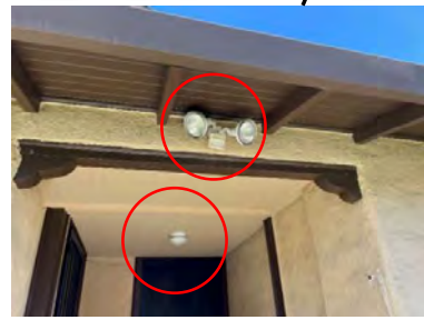
Phase: Design/Construction Comments: Adjust note. Floodlight and circuit to be removed. New compatible fixture to be selected at ceiling.
