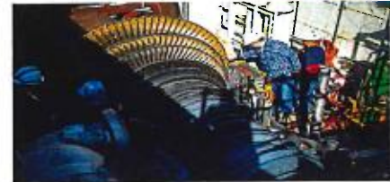
Steam Turbine Rotor Exposed
