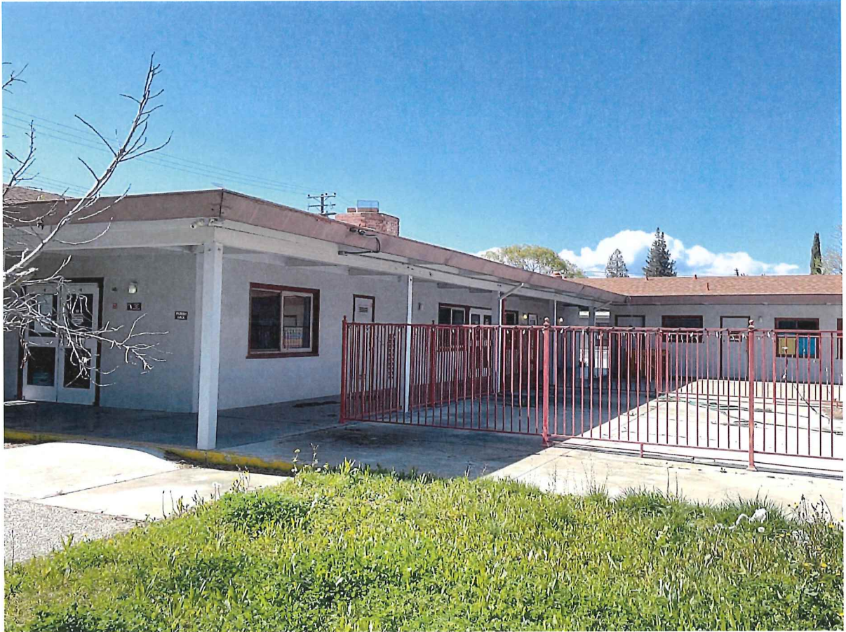
Photograph 15 1957 Pruneridge Avenue, Santa Clara View: Single-story admin building on the south side of the courtyard.
