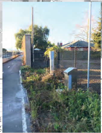
UTILITY BOXES NEAR SS MAIN
