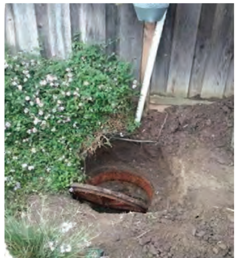
A C-2 MH 15-16 GROUND SURFACE
