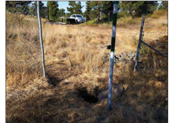
A C-44 MH 103-12 GROUND SURFACE
