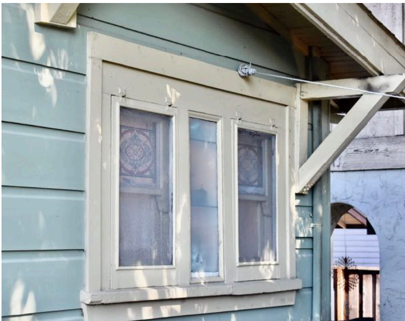
Three details of the rear addition: The paired vinyl doors (at upper left), a one-over-one window (at upper right), and a tripartite "ribbon" window (at left).
