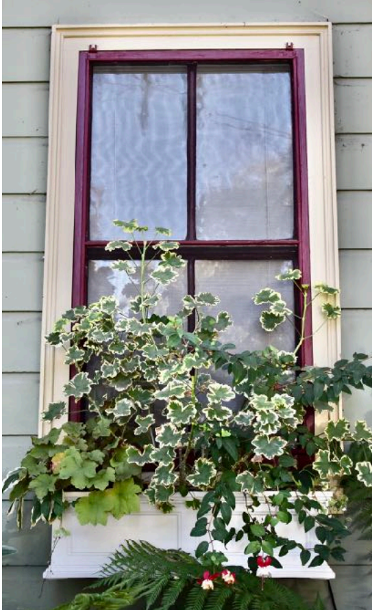
Below: Two-over-two window to the left of the porch (at left) and the nine-light window facing the porch (at right).
