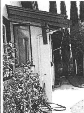
Left – Photo No: 100_2917 View: Front Porch roof trim; Photo Date: December, 2021 Camera Facing: SSE
