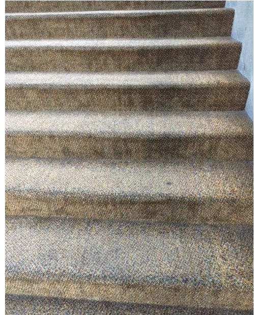
Figure 39: SCCC Carpet Condition
