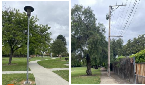
05 Park Lighting/Power Pole
