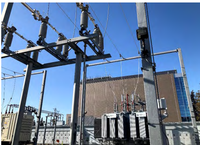
Fairview Substation Transformer
