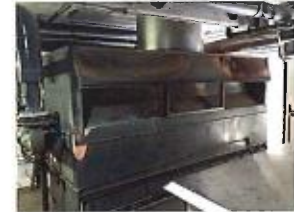
Swim Center Boiler
